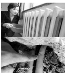
Heating Pipes/ Underfloor Heating Pipe Leaks
