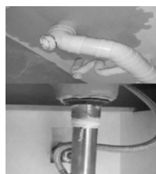
Water Supply Pipe Leakage/ Water Pipe Leakage
