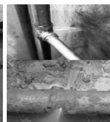
Fire Sprinkler System
