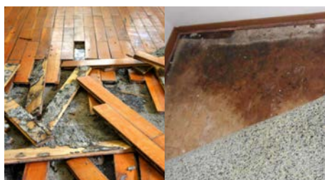
Leak Under The Floor
